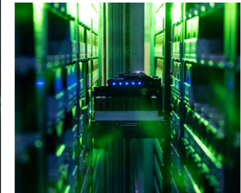
DATA STORAGE FOR THE CASCADE SUPERCOMPUTER AT CDC DATA CENTRE IN AUCKLAND
